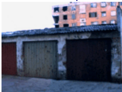
A closer view of some flats—that are still occupied and the bullets on the garage
